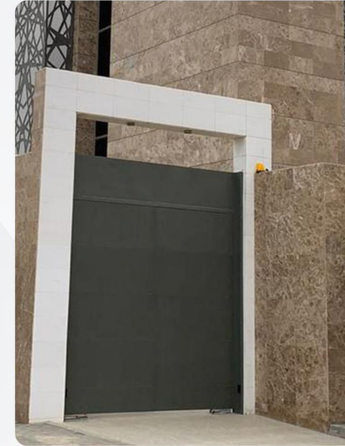
Supply and installation of natural stone for the exhibitions and offices project of Al - Khorayef Real Estate Investment Company - Al - Kharj Old Road- Riyadh
