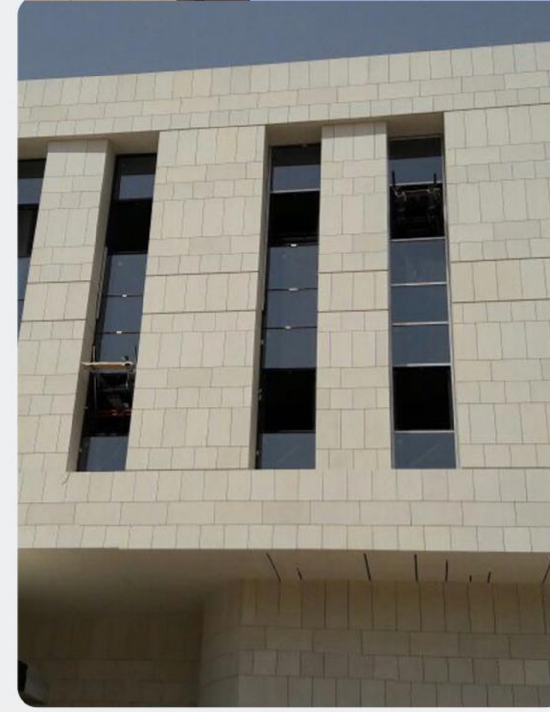
Supply and installation of natural stone for a residential commercial complex , Al - Bani Development Company – Al Dabab Street - Riyadh
