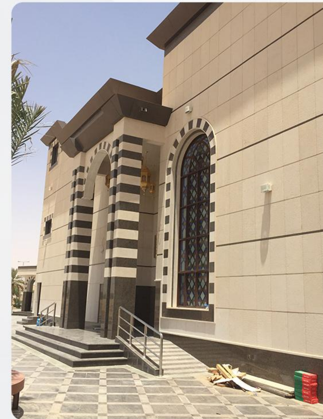
Supply and installation of natural stone , Al - Nasyan , Mosque Buraidah , Al - Qassim
